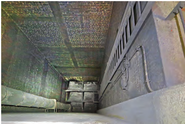
The view deep into one of the two vent shafts, coated in thick carbon pollution. Photo Clive Penfold
